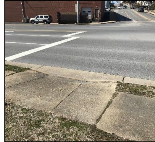
Uneven sidewalk surface on east side of the Hampton Street intersection
