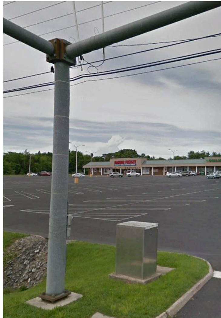
Figure 31: Existing Outdated Signal Equipment at US 250 and K Mart/Big Lots Business Entrances
